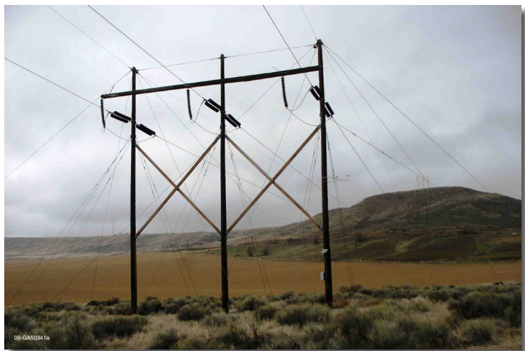
INL research on how wind cooling affects high-voltage power lines aims to increase transmission capacity at very little extra cost.
